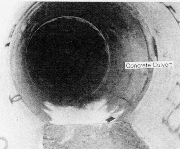
Photograph 11. View looking at a track station located within the upper concrete culvert north of the 210 Freeway and in close proximity to Drainage 4. Although evidence of coyote use, including scat was observed on the access road leading from the 210 Freeway to Drainage 4, no evidence of movement was detected at this station or anywhere within the concrete culvert.
