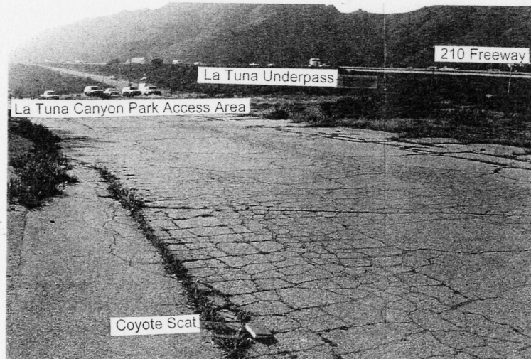
Photograph 16. View looking northwest along the La Tuna Canyon Park access road located immediately west of the La Tuna Canyon Road Underpass. Note the coyote scat in the foreground.
