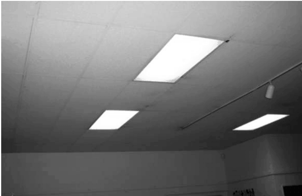
Typical Condition Of Flourescent Lights
