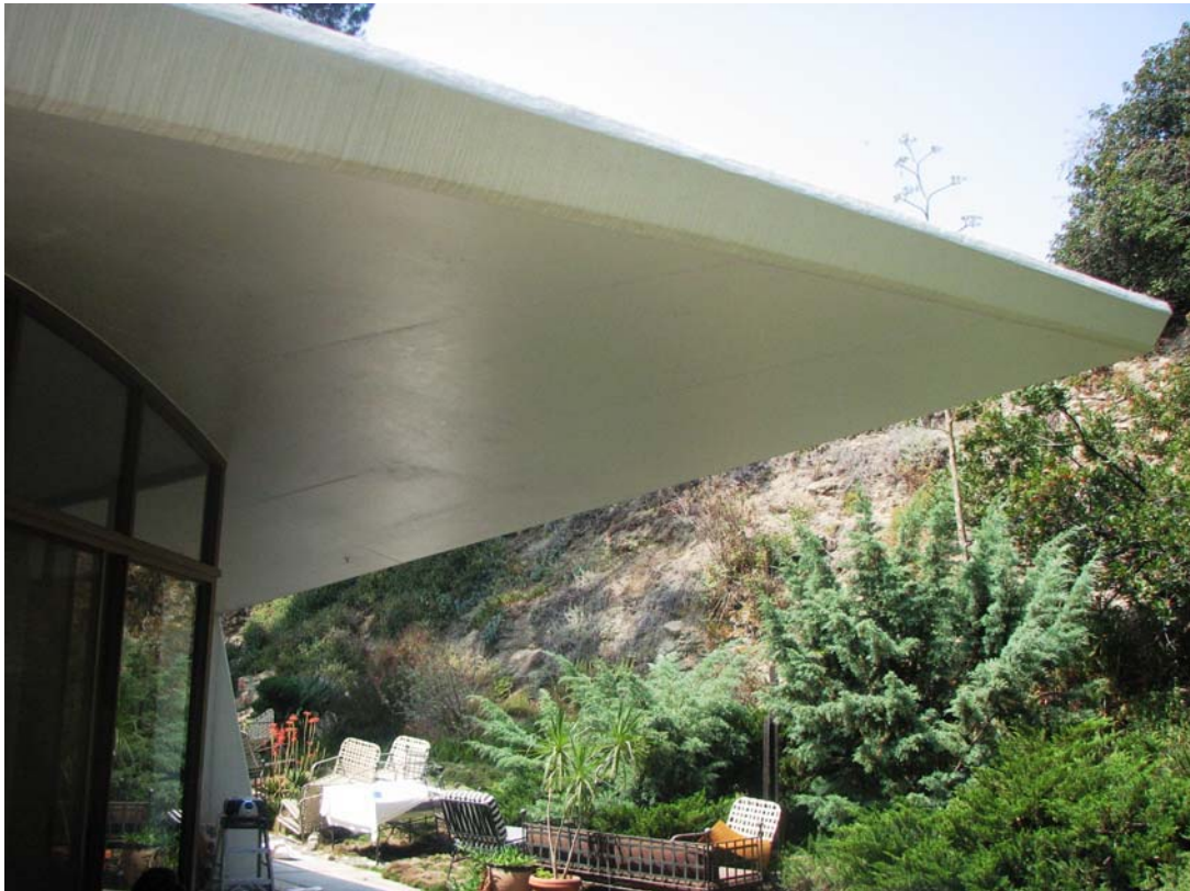
James F. Real Studio-Office, roof overhang, 77 Patrician Way (Photograph by Charles J. Fisher)
