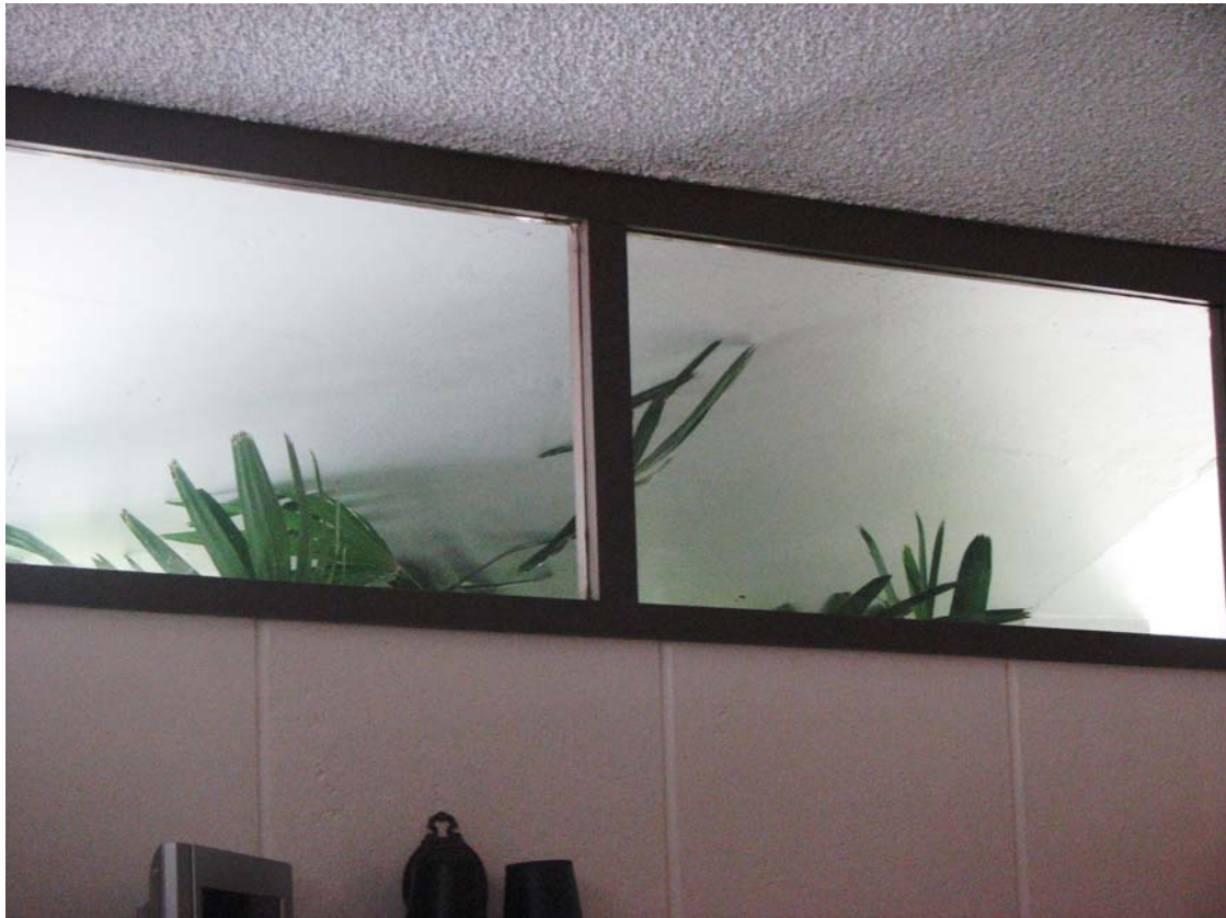
James F. Real Studio-Office, clerestory windows, 77 Patrician Way (Photograph by Charles J. Fisher)
