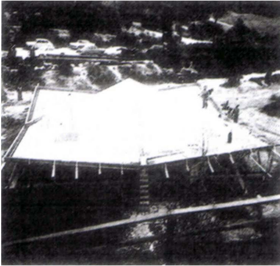
James F. Real Studio-Office, freshly poured concrete roof (Pacific Bridge Company photo))
