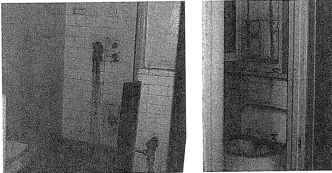
Interior of a typical bathroom before the construction, pictured tile contained lead (2008)
