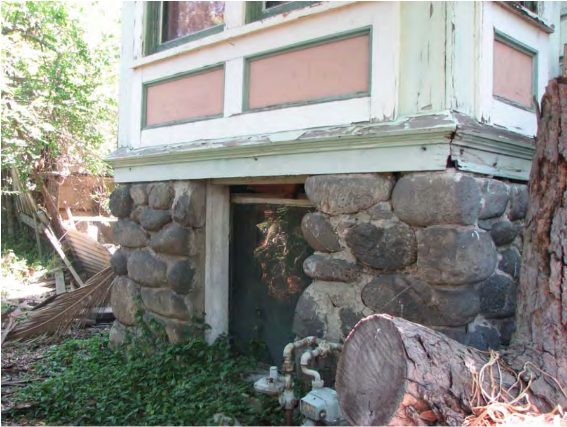
Young-Gribbling Residence, stone foundation, 3320 Griffin Avenue, July 1, 2011 (Photograph by Charles J. Fisher)
