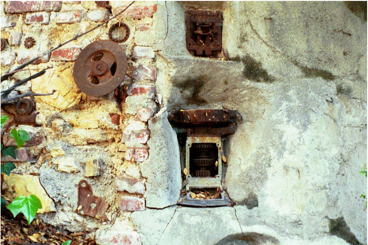
Hermon Car Wall, 400 Block of Pullman Avenue (Photograph by Charles J. Fisher)
