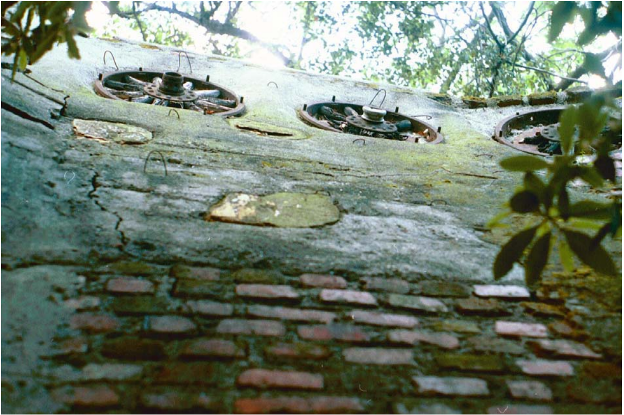
Hermon Car Wall, 400 Block of Pullman Avenue (Photograph by Charles J. Fisher)
