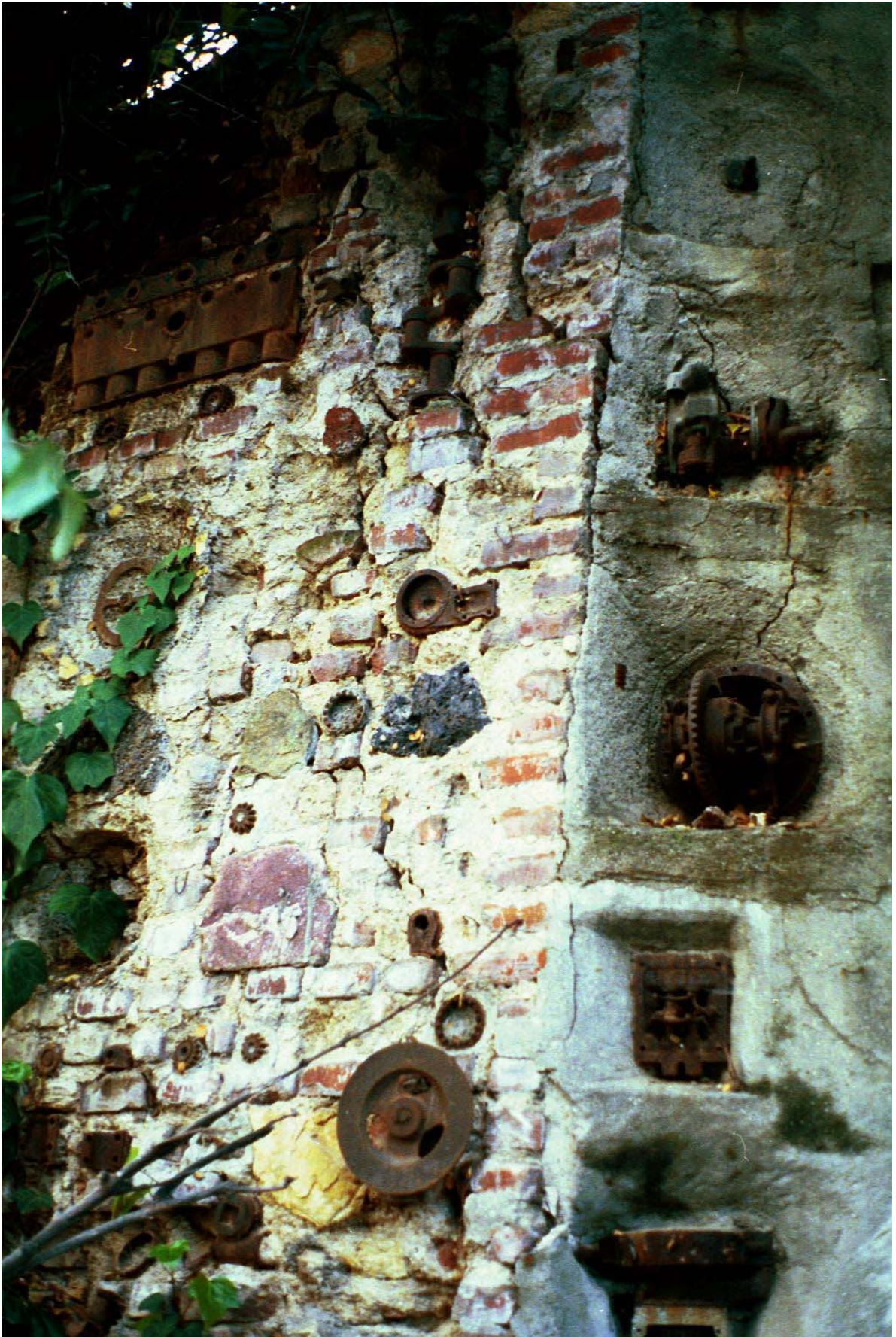
Hermon Car Wall, 400 Block of Pullman Avenue (Photograph by Charles J. Fisher)
