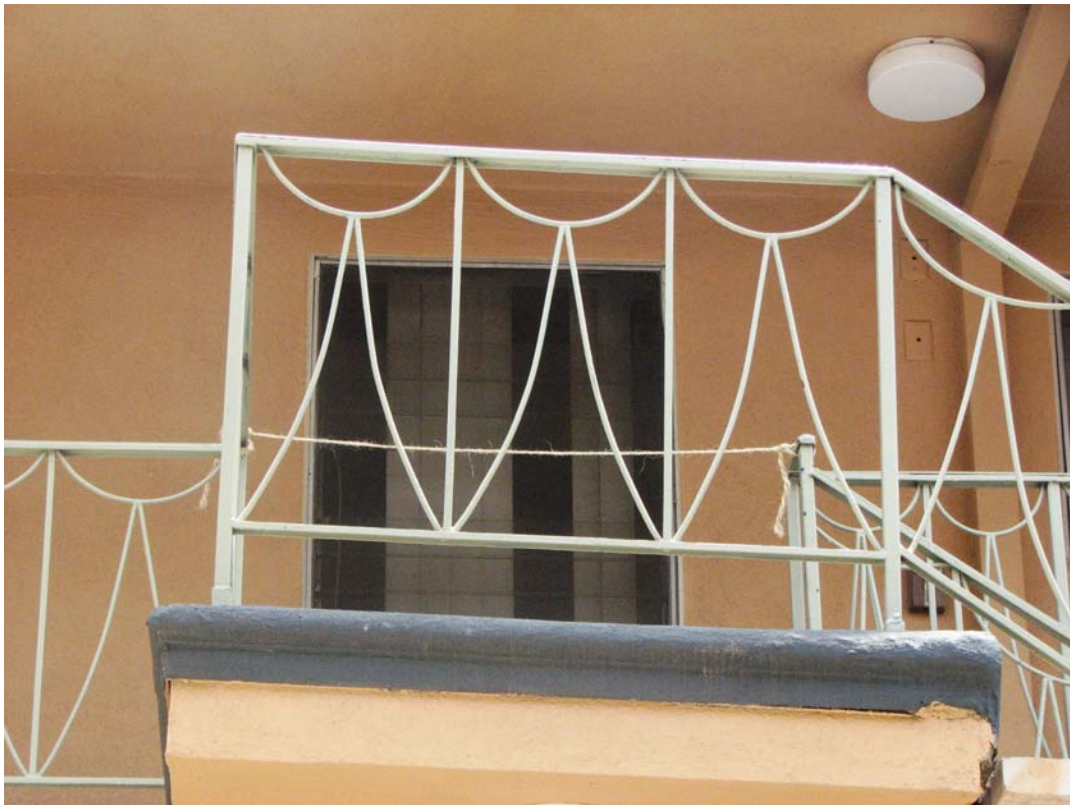
The Ardmore Wilshire, stair railing, 722 S. Ardmore Avenue, July 4, 2008 (photo by Charles J. Fisher)
