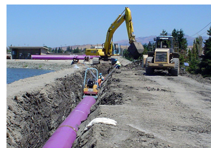
Purple Pipe for Recycled Water
