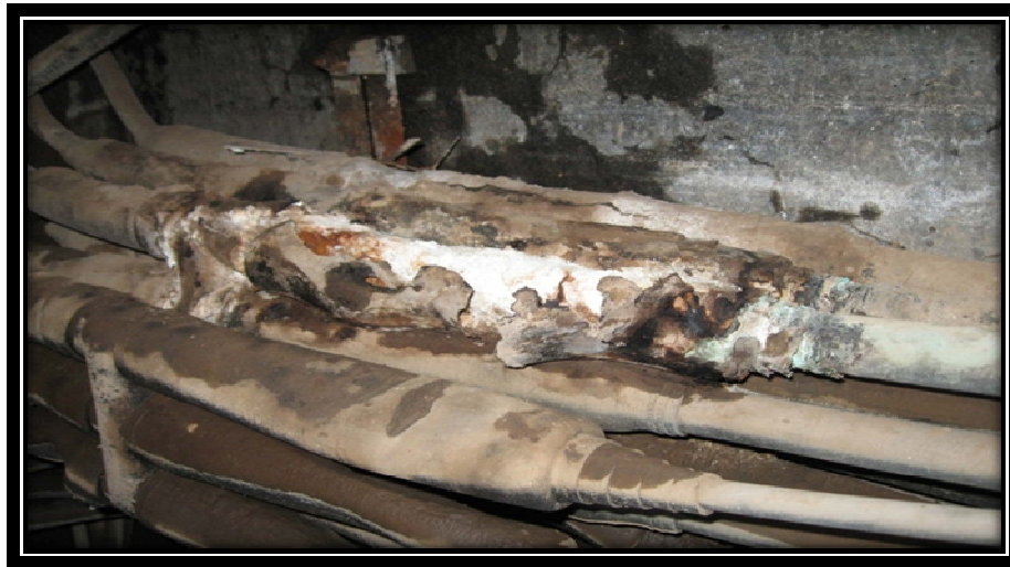
Picture: Illustrative of Cable Scheduled for Replacement.
