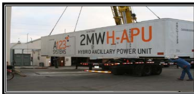
Figure K-2. Lithium-ion batteries.
