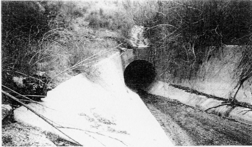
Photograph 7. Beginning at the confluence with Tributary 4.5, Drainage 4 exhibit surface water flow, which continued to the culvert that extends beneath Interstate 210
