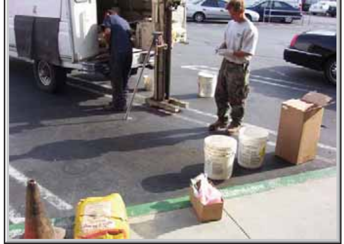
View of drilling the front exterior Boring #3 at the Victory Plaza Cleaners.
