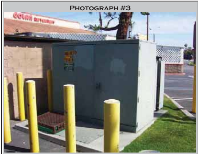
View of a pad-mounted transformer.
