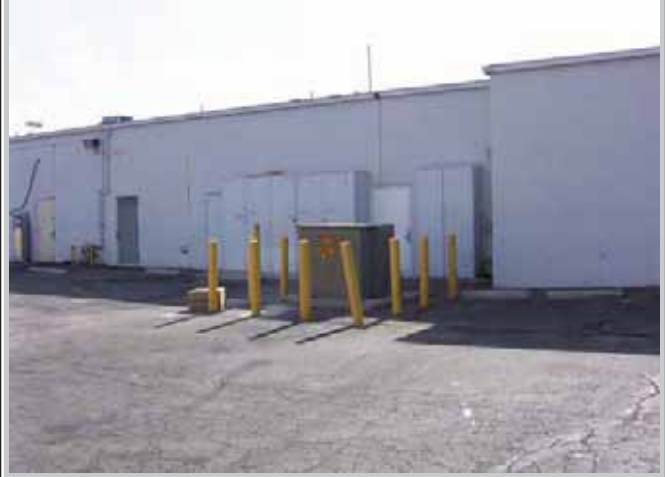
View of a pad-mounted transformer.
