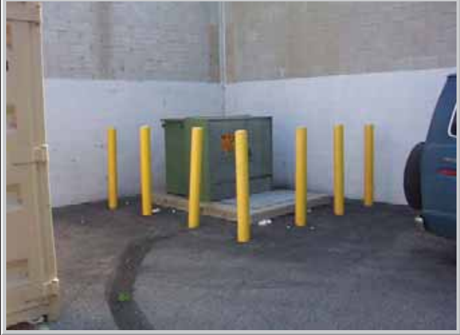
View of a pad-mounted transformer.
