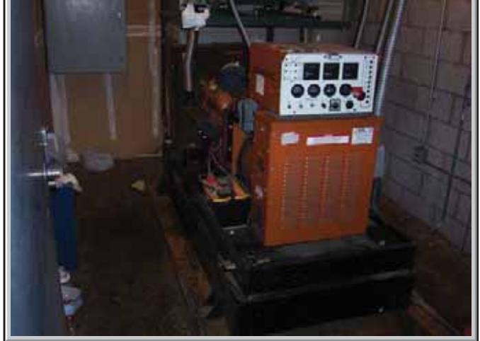
View of the backup generator at Vallarta Supermarket.
