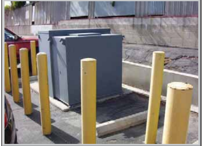
View of a pad-mounted transformer.
