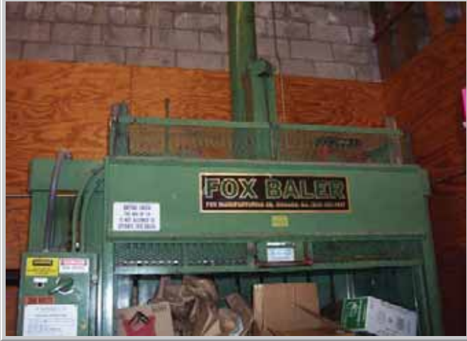
View of the compactor in the Vallarta Supermarket storage area.
