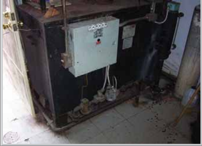
View of the dry cleaning equipment.
