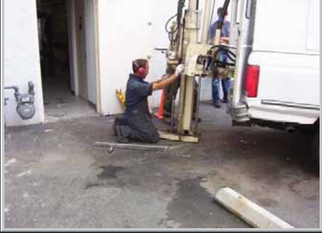
View of drilling the rear exterior Boring #2 at the Victory Plaza Cleaners.
