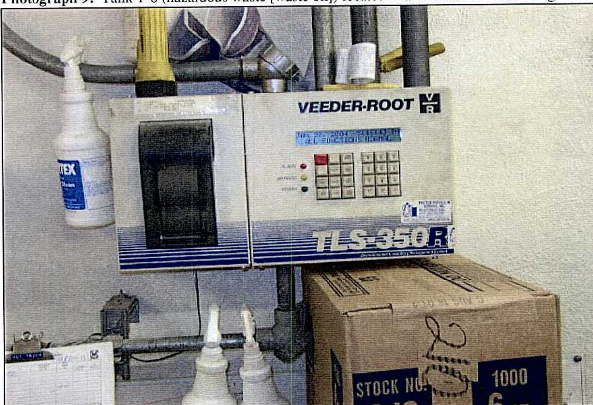
Photograph 10: UST monitoring system control panel.
