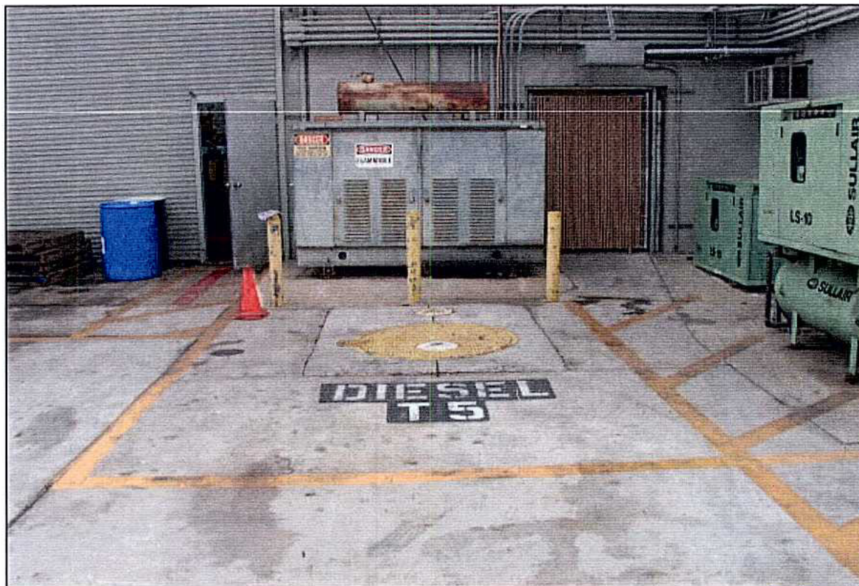
Photograph 7: Tank T-5 (diesel UST) and emergency generator located on south side of tire station area.
