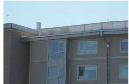
Metal screens could be utilized to hide utilities located on the rooftop. (Figure A.4.l)
