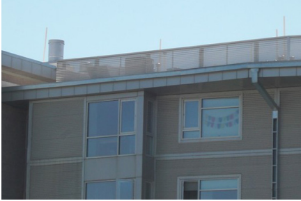
This screen hides the mechanical equipment on the rooftop of the building. (Figure A.3.p)
